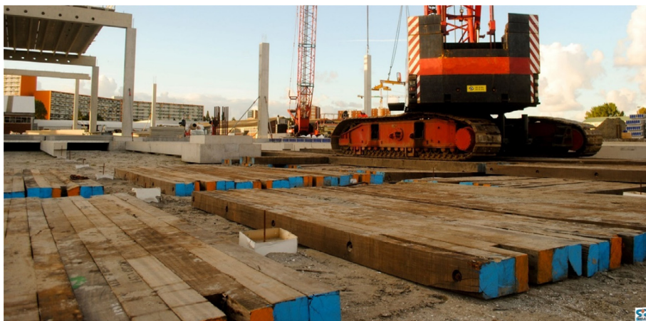
FIGURE 7 Crane mats in use at a building site (photo by courtesy of Welex).
